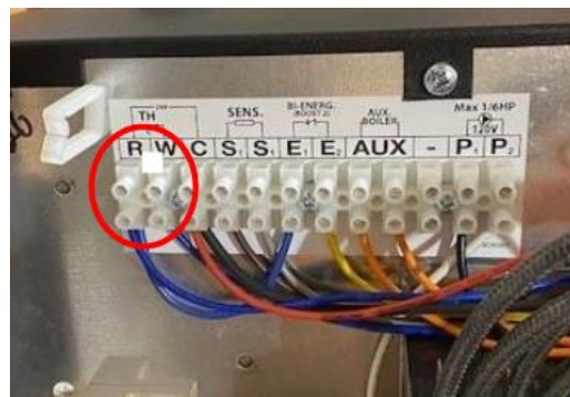
Back Up Terminals on Boiler
