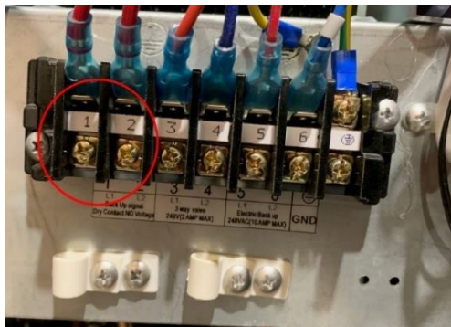
Back Up Terminal on Heat Pump
