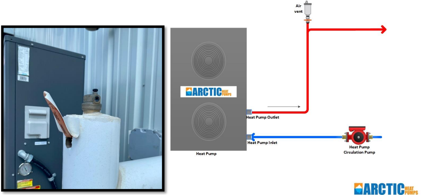
Typical air vent installation with insulation and shut off valve on the outlet line of the heat pump.
