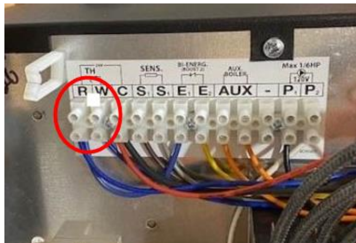
Back Up Terminals on Boiler
