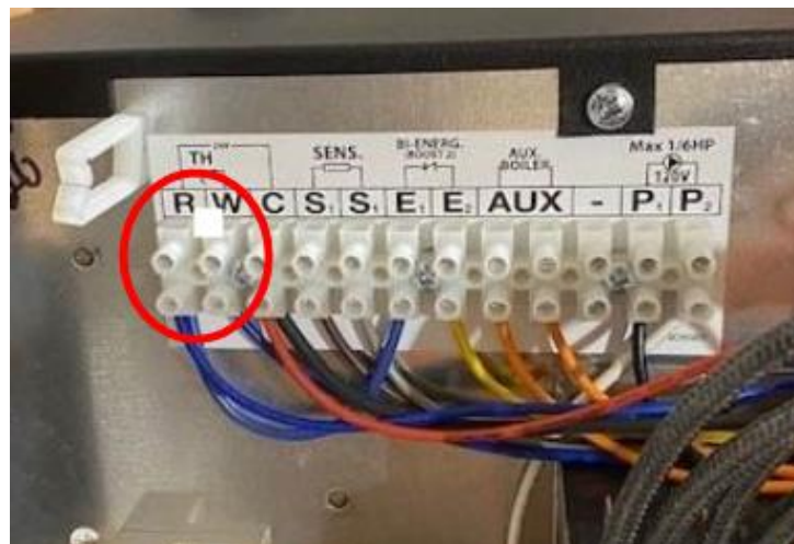
Back Up Terminals on Boiler
